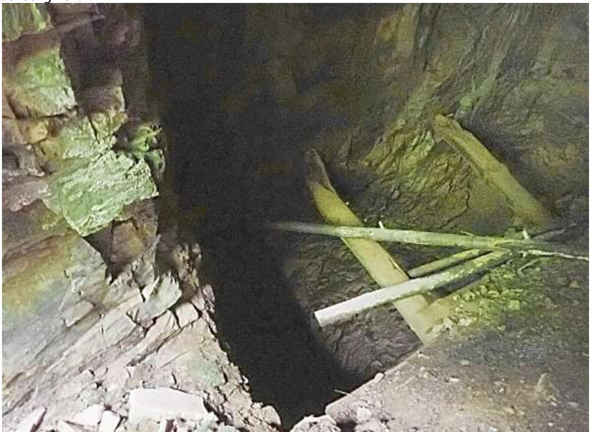
Photograph 21. Exposed open stope looking down to lower level (timber props support the walls).
